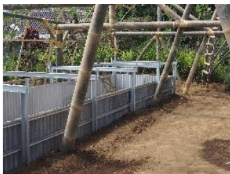
Figure 5. Hydroponic Installation (6 days)
