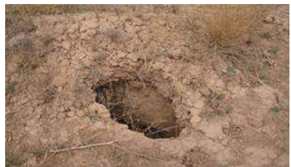
Fig 7. Hole in the gully
