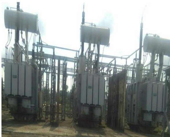
Figure .3 Three Single- Phase Transformer in Thanlyin Primary Substation
