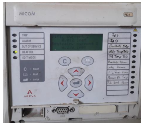
Figure.5 Differential Relay using for Thanlyin Substation
