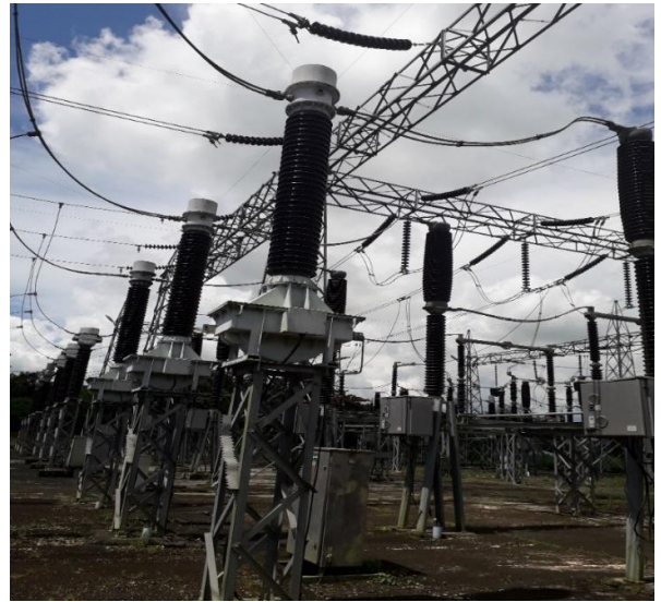
Figure.4 Current Transformer for 230kV side
